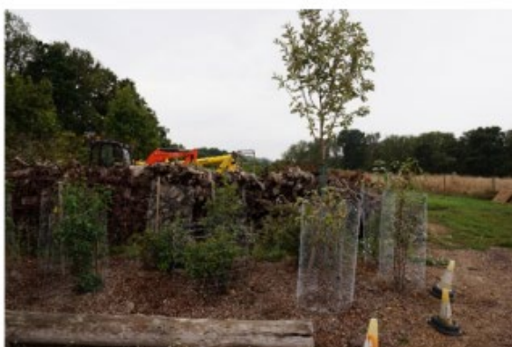
Showing wooded backdrop to parcel and tree planting taking place at time of the survey
