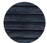
Black stained Weatherboard
