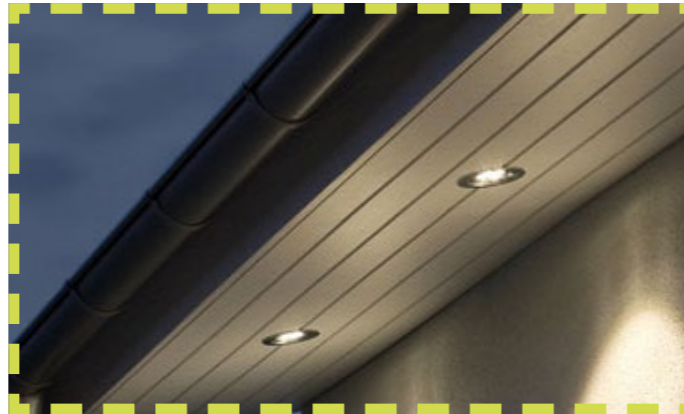
Light fittings attached to pavilion
