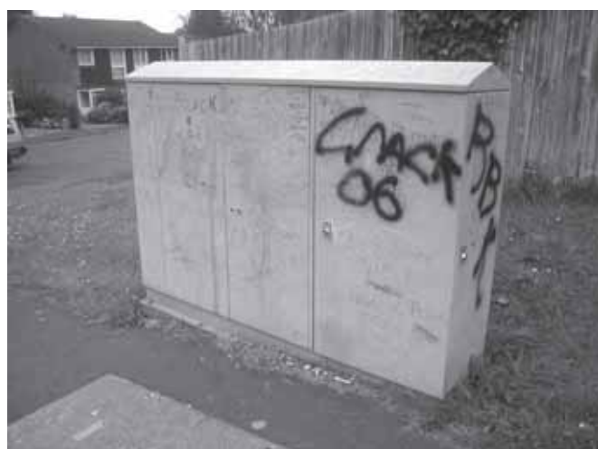
Junction box with graffiti on verge
