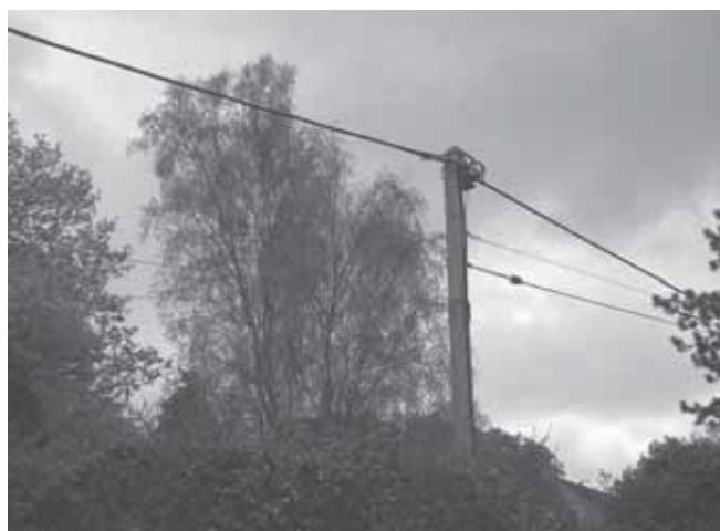
Overhead cables in Halterworth Lane
