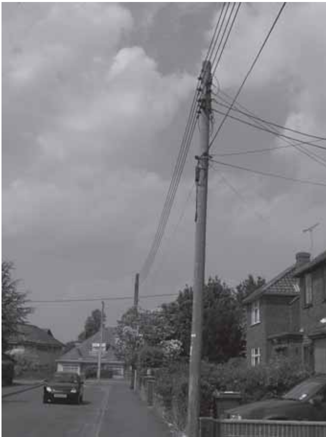
Electricity feeder poles and cables
